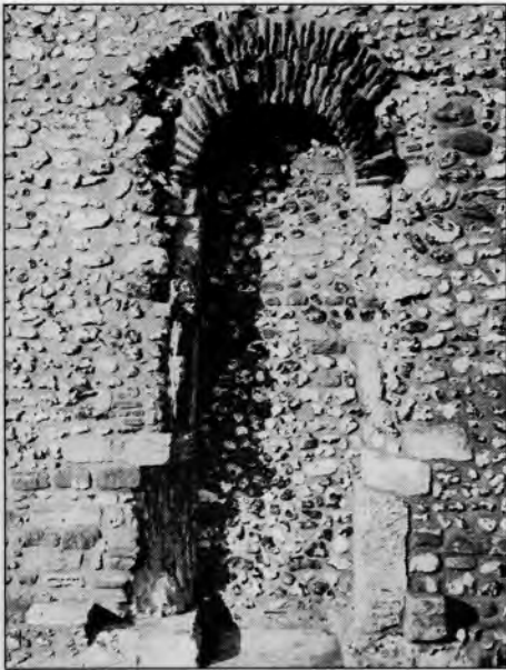
The old Saxon south door as it is today after being excavated and exposed to the elements since the 1860's.
